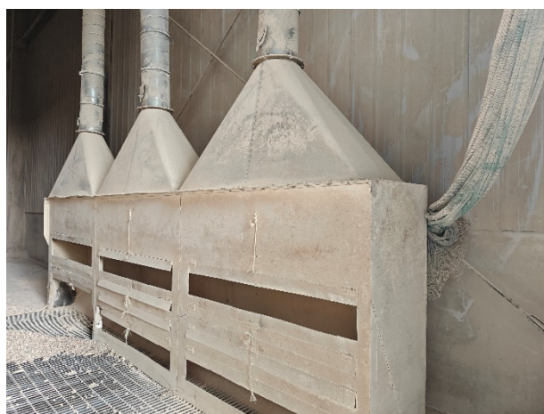
卸料车间抽风口
